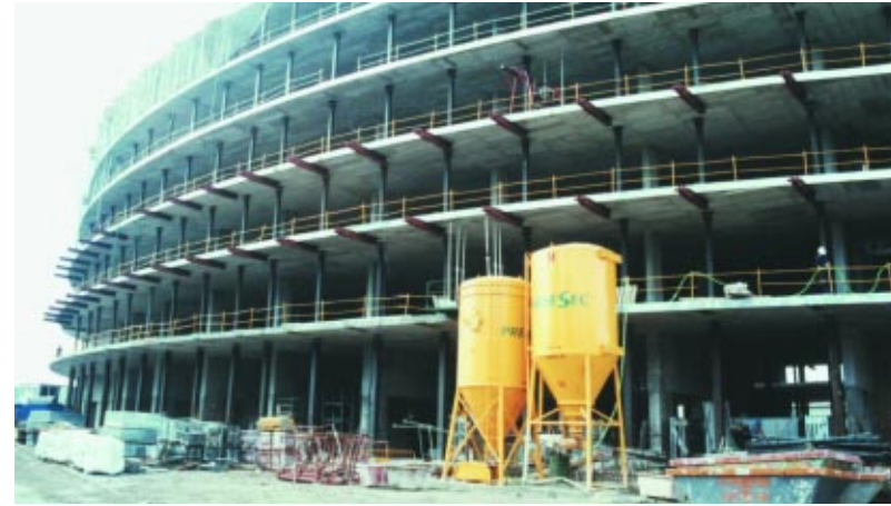
3. HEB 300 props each of which are 3.6 m below the internal braces of sectors II and III. 4. Interior of sector I propped. 5. Decks propped up every 3.6 m during the construction phase.
