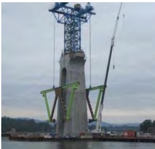
Figure 19. View of the erection of the zero “W” steel segment over one of the central piers
