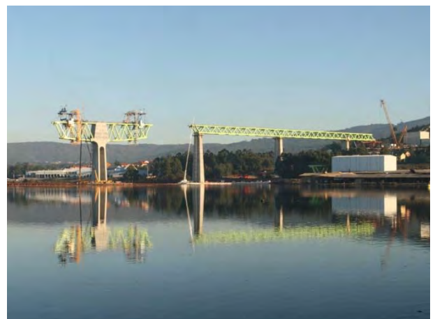
Figure 20. View of the current state of the works near abutment A1 (December. 2013)
