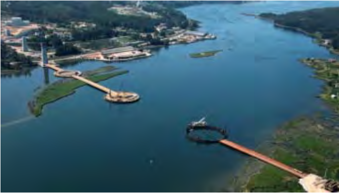
Figure 18. Aerial view of the construction of the foundations of the three central piers
